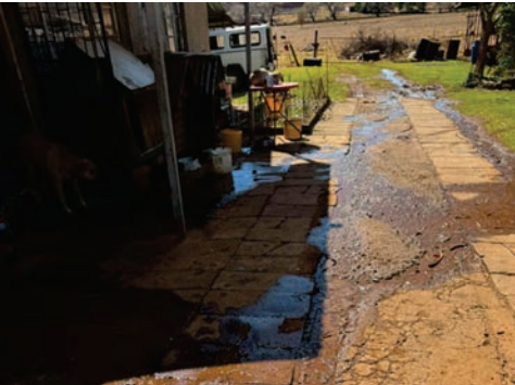
Sewage spilling into a yard in Groenvlei.
