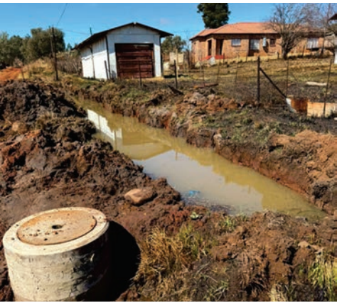
The sewer ditches that were dug and left open in Groenvlei.
